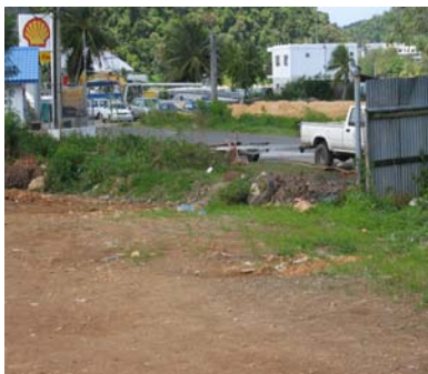
Part of landfill not gated or fenced
